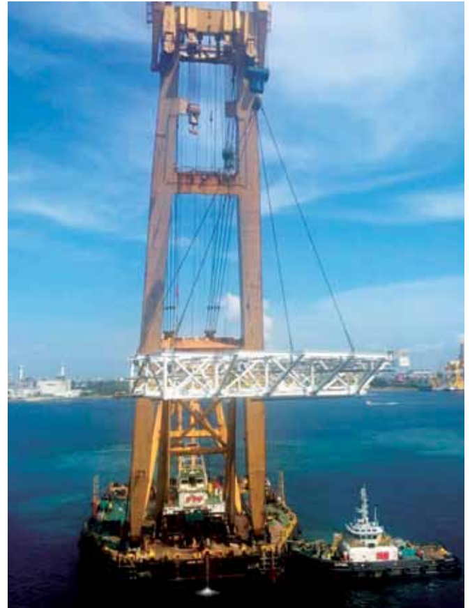
11 May 2015: After the installation of the two blisters, the Helideck Truss was lifted onboard
