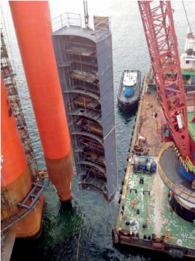
10 May 2015: Within three weeks from the first project meeting on 22 April 2015, Keppel FELS had designed, fabricated and lifted into position the two blisters
